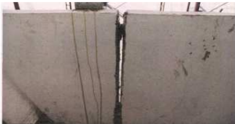
A gap in a wall at the klia2 building. The airport's project manager and main contractor have failed to obtain a Certificate of Completion and Compliance for the terminal building.
